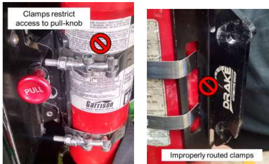
Figure B-45: Incorrect orientation of extinguisher clamps.
